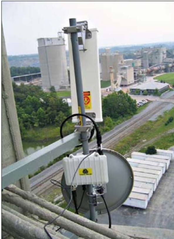
Figure 4 2.4 GHz sector and 5.8 GHz backhaul dish antenna
