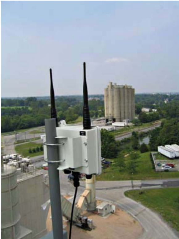
Figure 3 Wave Relay™ installation.
