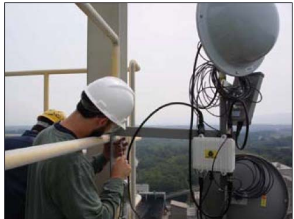
Figure 2 Installation of sector antennas and wireless router.
